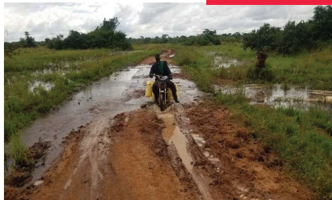
A Section of Gomero, Migani, Kagongi, Buwana community access road in Nakaseke before it was rehabilitated under the LEGS Project.
