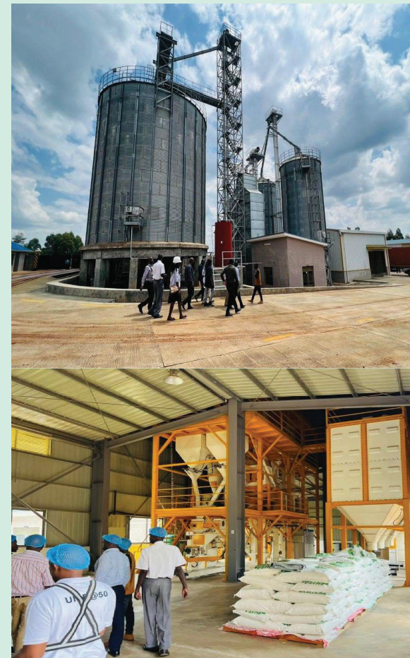
(Above) Installed 1000 metric tons (Silos) (below) The maize processing and packaging component.
