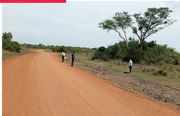
The 33 Km access road from Gomero, Migani, Kagongi, Buwana in Nakaseke District after it was rehabilitation by the LEGS Project in December 2022.
